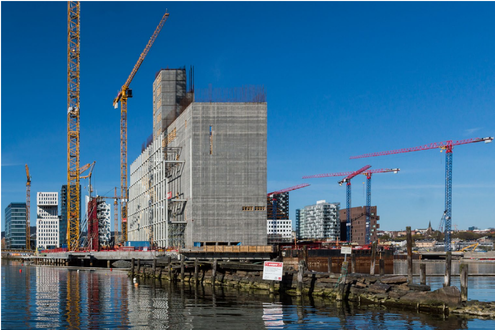
Figure 7. Lambda under construction. Seen from the south side on 1 May 2017. The Barcode buildings are in the background. Source: Aleksander Bern.
