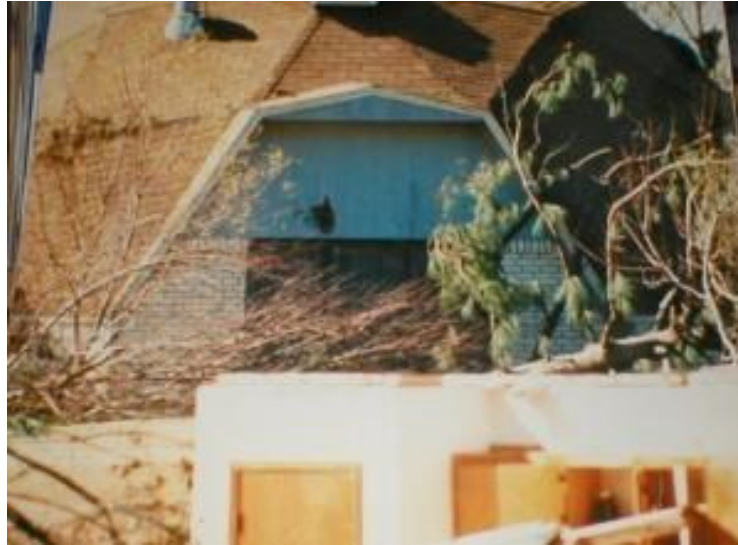
Figure 2.13: A dome hit by a tornado in Jacksonville Texas (AGE Dome)
