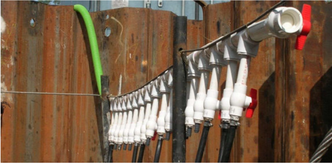
Figure 5.17 WB I-80 Bridge cooling pipe system manifold
