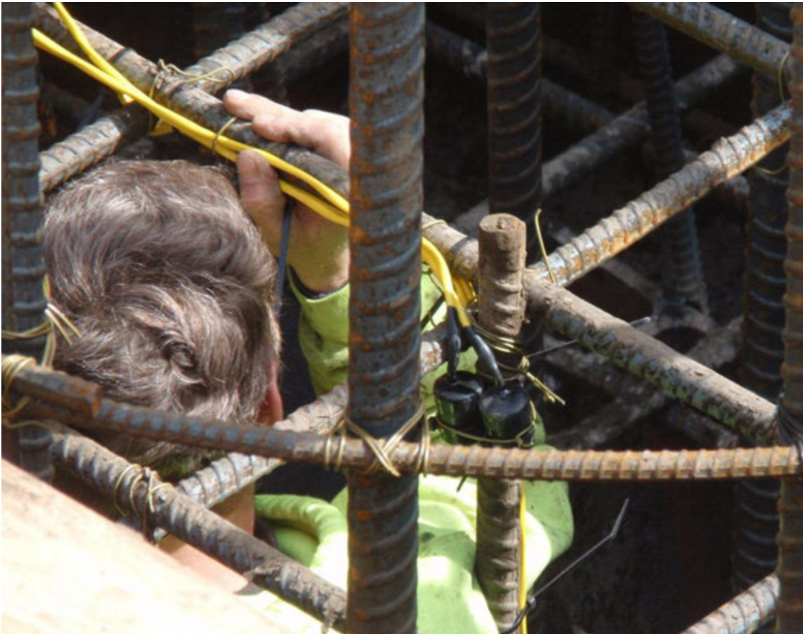
Figure A.1 Installation of thermal sensors with cable ties and tie wire
