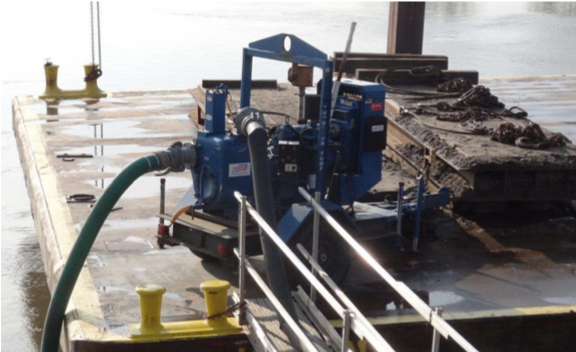
Figure 5.15 US 34 Bridge cooling pipe system water supply pump
