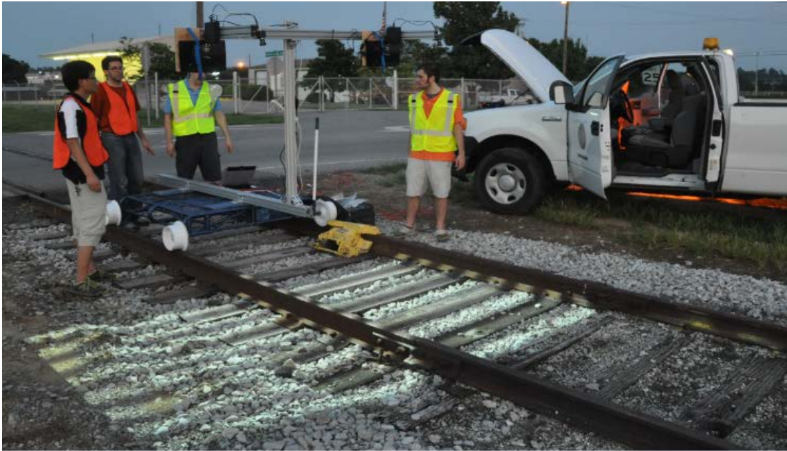
Figure 3.3 Field Test at crossing (USDOT 719862A) on Beasley Road, Versailles, KY.
