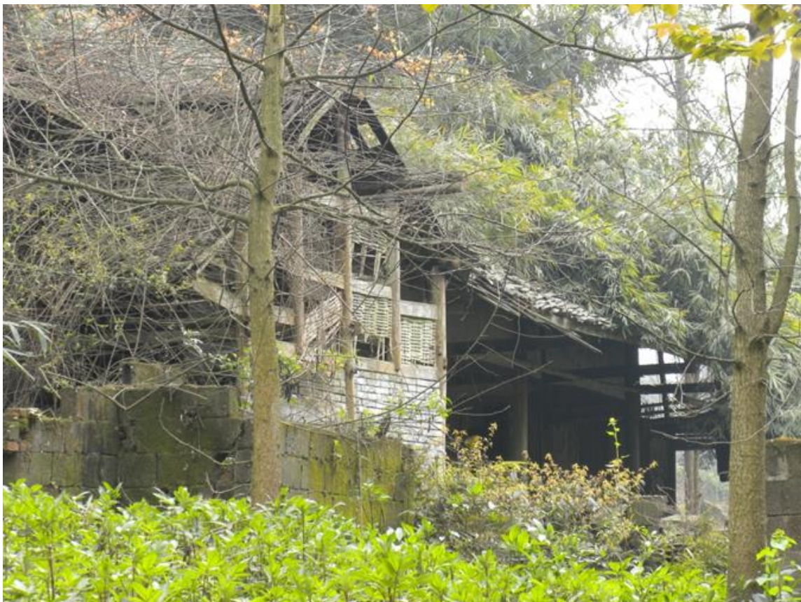
Figure A.3.84. Earthquake Damage to a Chaping Resident of a Rural Community
